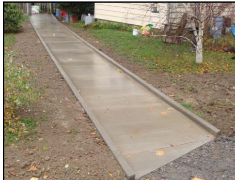
Above: ATI installed a sidewalk to provide access from an individual's driveway to their home entrance.
